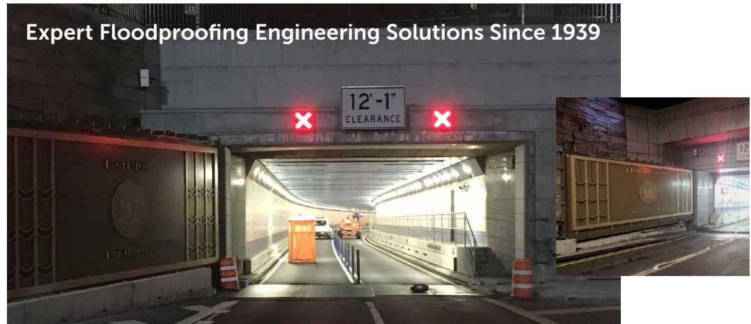
Flood Gates Protecting NYC Queens Midtown & Hugh L. Carey Tunnels From Flooding
