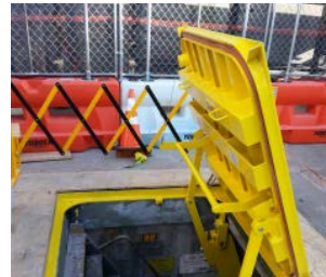
NYC Emergency Egress Hatch
