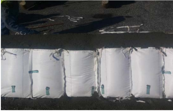
Connected 2' x 4' VersaShield Filled With Sand
